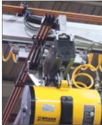
Electric supply using Insul-8
